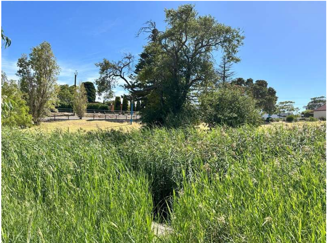
Figure 3. Existing stormwater outfall that needs upgrading + potential deeper, open/low-reed pool
